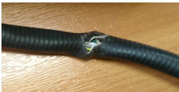
Figure 13. Damaged wire protector.
